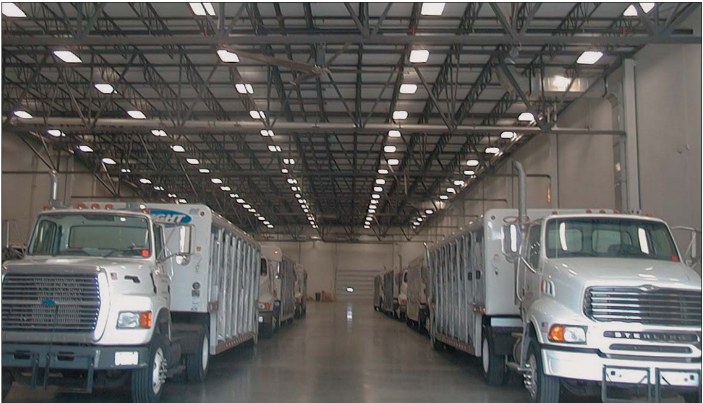
Two 24' HV/LS Revolution Fans were installed to help keep College City Beverage employees comfortable.
